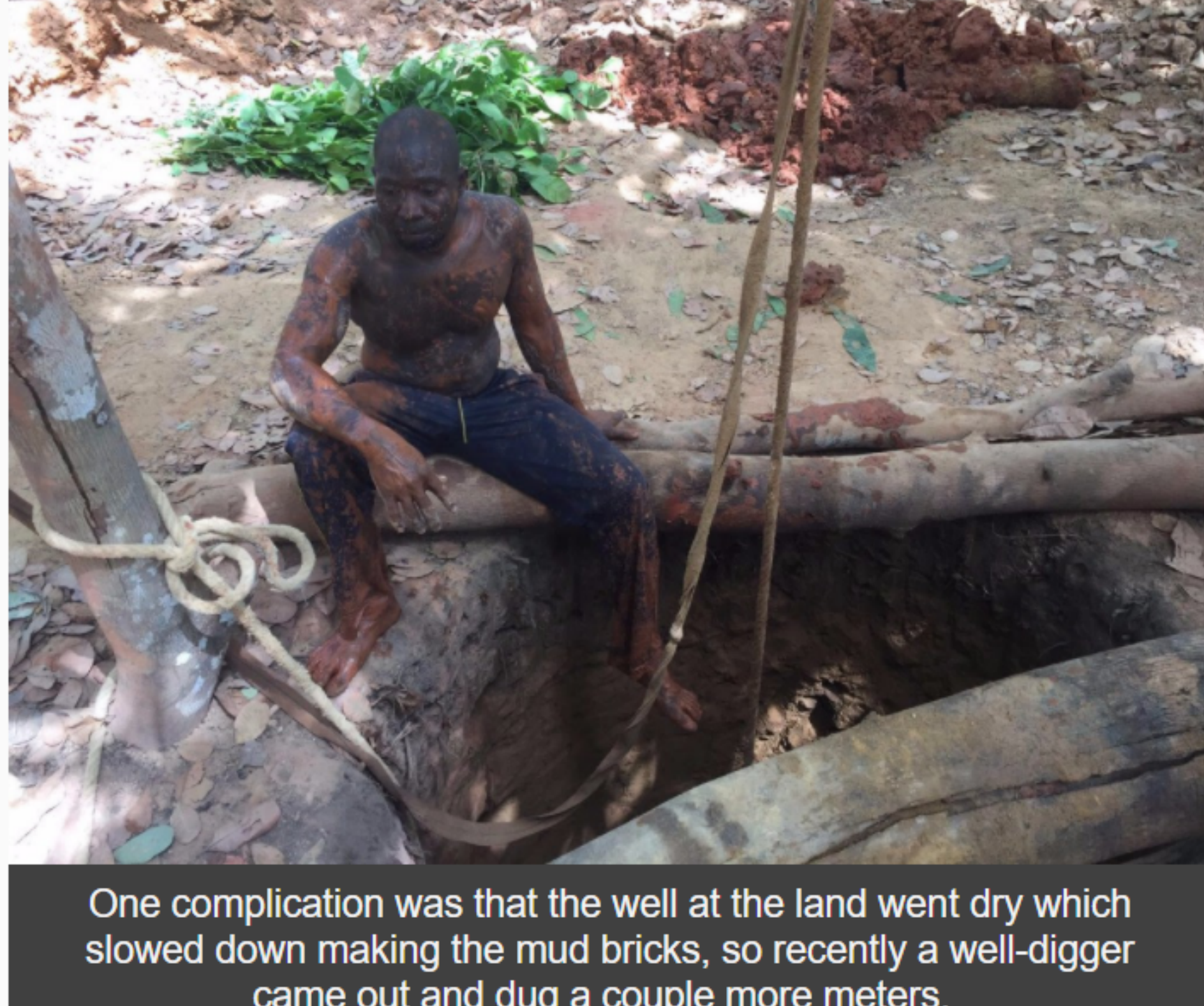
One complication was that the well at the land went dry which slowed down making the mud bricks, so recently a well-digger came out and dug a couple more meters.
